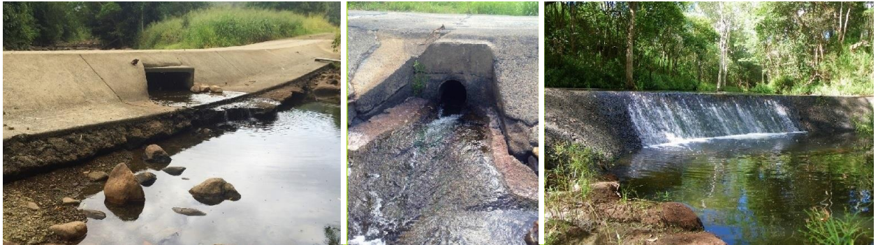
Figure 4. Left to right: Culvert causeway displaying a water surface drop, shallow water surface (through culvert and on apron) and velocity barrier (during medium- high flow conditions) exacerbated due to a culvert diameter <60% of stream width; Pipe causeway displaying velocity and behavioural barriers (insufficient lighting in pipe) and water surface drop barrier.
