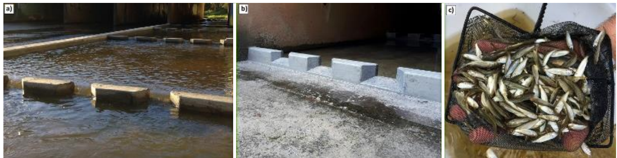
Figure 16. a) Retrofitted horizontal culvert baffles in operation under Paradise Road on Slacks Creek in South-east Queensland. Note: Nib wall on left hand side to divert all base attraction flows down the fishway. Prior to remediating this barrier, the flow was spread out across four 2.4 m wide culvert barrels creating a shallow water surface barrier under base flow conditions. b) Horizontal baffles with the boxing recently removed c) Predominantly showing Juvenile sea mullet and striped gudgeon captured successfully ascending through the horizontal culvert baffle fishway at catch rates of 256 and 793 individuals per day respectively.
