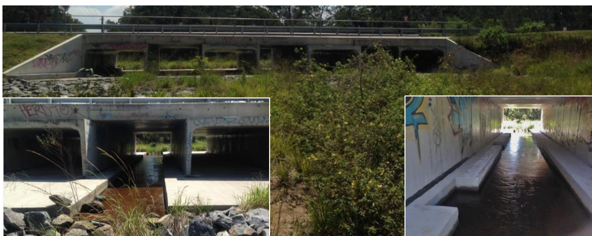
Figure 11. Culvert crossing conforming to Accepted Development requirements. Note: Low flow channel and wall roughening.
