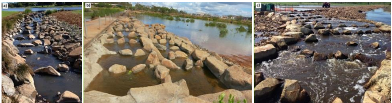
Figure 12. Nature like rock-ramp fishways: a) Full width (Gooseponds Ck, Mackay), b) Dog-leg (Lake Callemondah, Gladstone) c) Partial width (Tedlands Ck, Koumala)
