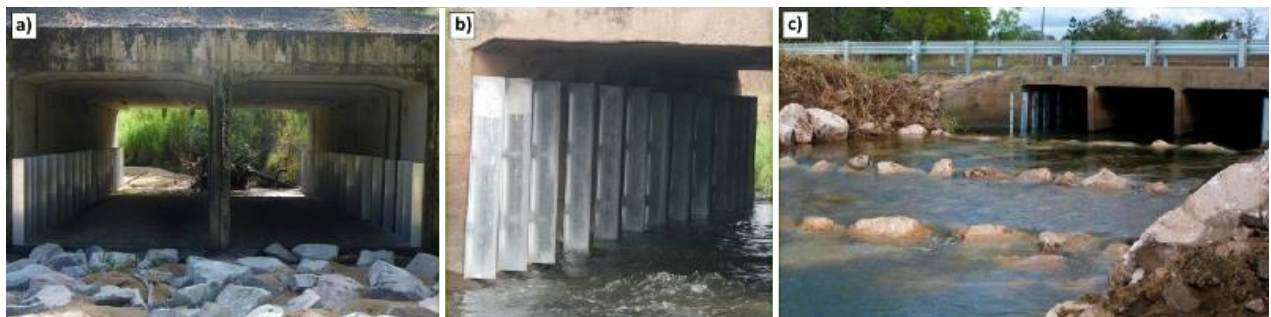
Figure 15. a) Vertical culvert baffles with scour protection (Aims Rd, Townsville) b) Close up view of vertical baffles retrofitted to a culvert c) Vertical baffles in conjunction with a rock-ramp fishway (Sheepstation Creek, Ayr).
