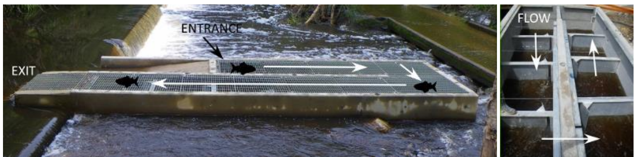
Figure 14. Showing a vertical-slot fishway on Waterpark Creek, Byfield. Note: The partial-width nature and small entrance of vertical-slot fishways makes it difficult for fish to locate the entrance.
